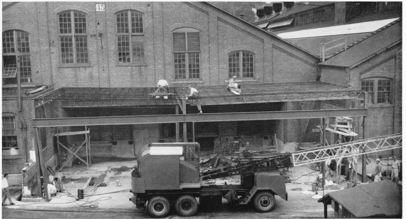
Construction of the new truck well at the North Mill called for a special hoist (foreground) which was imported from the Berlin Construction Co. in Berlin, Conn. to hoist and place the heavy iron work needed on the well.
